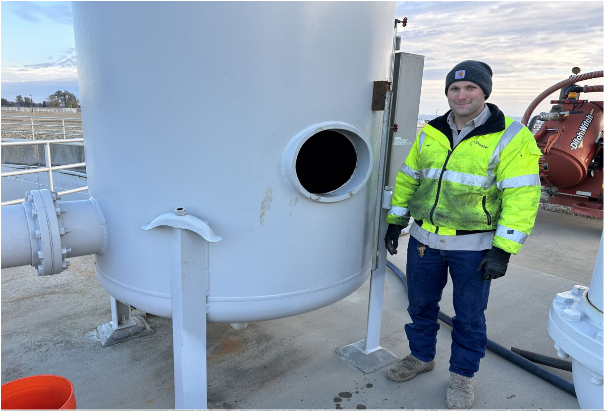
Photo 3&4: DAF Pressure Tank #1 outside and inside.
