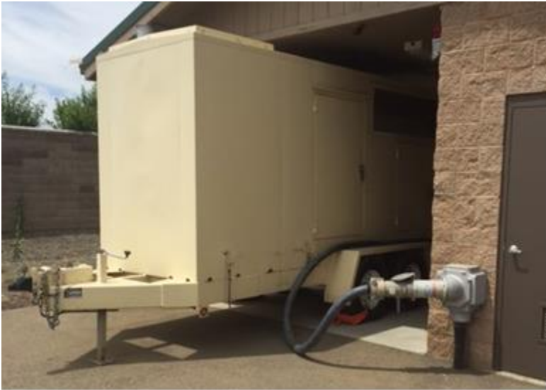
One of the City's diesel-powered generators
