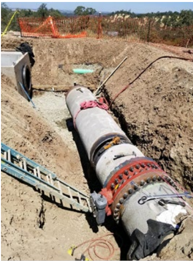
Connection of 36-inch supply pipe from metering station to Tank 3. Butterfly valve in foreground and altitude valve vault at back left.
