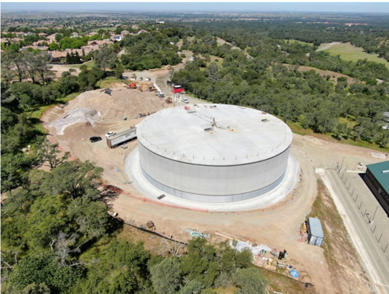
Looking northwesterly at the tank with the metering station to the right. The steel tensioning cable (visible at the base of the tank) is being applied from the bottom to top. The red cab of the wrapping machine can be seen circling around the back of the tank.
