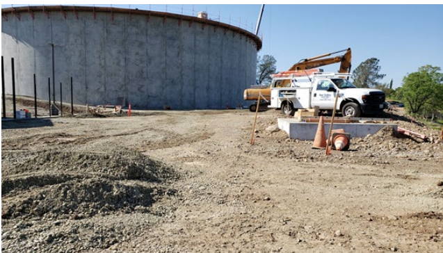
Looking west at the completed tank. Workers are removing falsework and formwork by crane through hatches in the roof.
