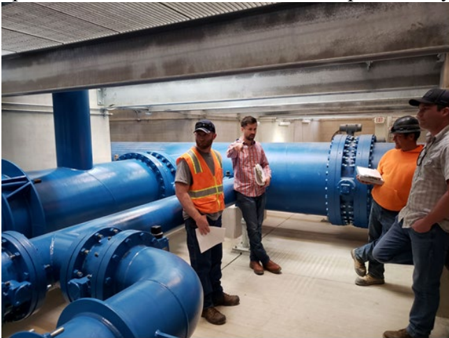
View from the pipe gallery (basement) showing 16-inch and 42-inch pipelines that will serve the City of Lincoln.
