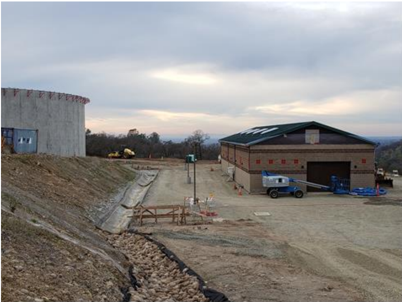
Northwesterly view of the Metering Station. The building is done, and the site is almost ready to pave. The City’s new 5MG Tank #3 is on the left.
