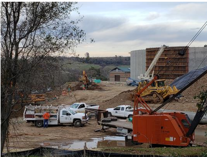
Looking east at Tank #3. Crews are installing the last of yard piping going into the tank. The last wall form on the tank is being removed. New PCWA Metering Station in the background.
