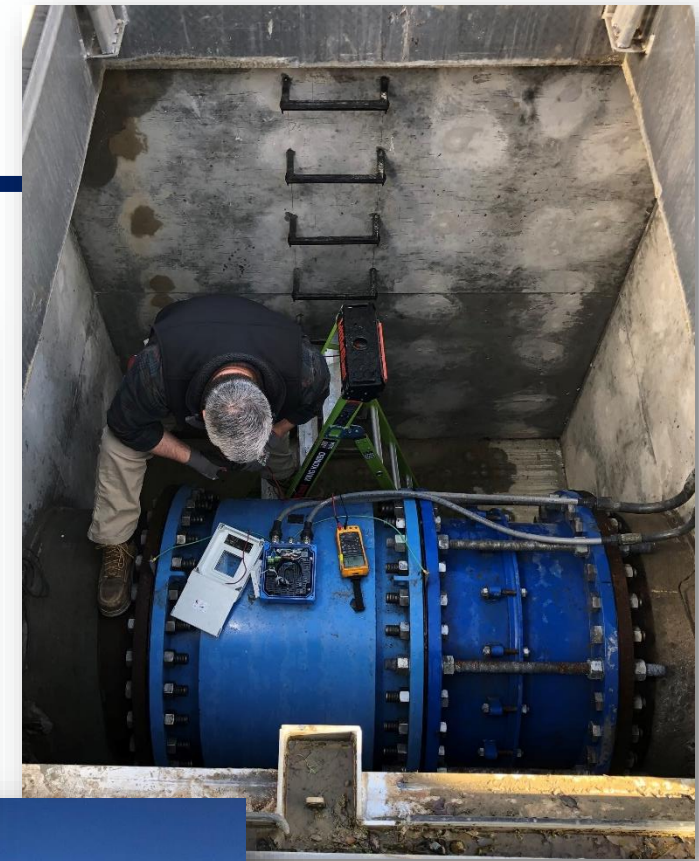
Large water flow meter leaving water storage Tank 3
