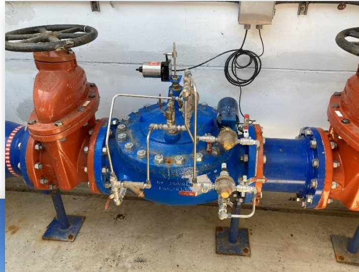
Pressure Reducing Station to ensure pressure zones are maintained
