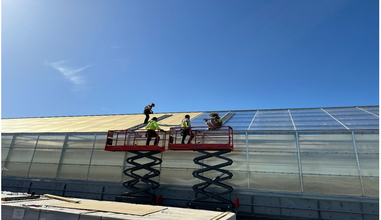
Photo 1. Greenhouse roof repair begins. Note the difference between the new and old panels.
